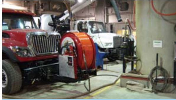
Vactor/Guzzler saves thousands of gallons of water for each truck that it tests by recirculating water from a holding tank (shown above) instead of using potable water from a spigot.
