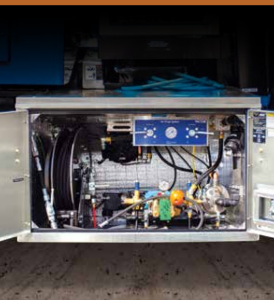
Water System Cabinet
